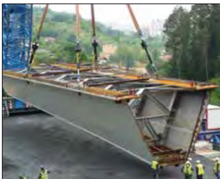
▼ Bridge segments are hoisted from the ground, being positioned with a 4-point SyncHoist system with fully monitored cylinders.
