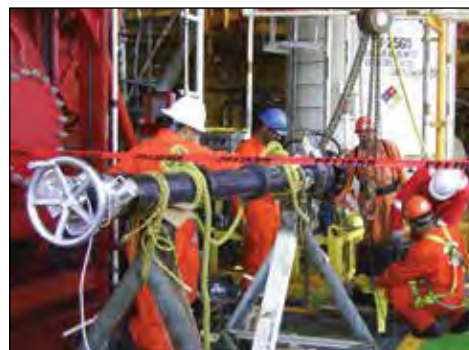
▼ CHT2000 hot tapping offshore application.
