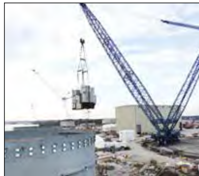
▼ Rigging engineers used the SyncHoist system to precisely monitor and adjust each lifting point independently, or together in a synchronized manner to position the 1140 ton nuclear plant module.
