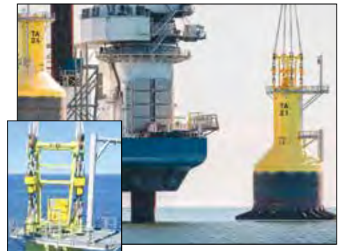
▼ Offshore wind turbine base foundations installed with a wireless SHAS-SyncHoist System to ensure the foundation remained vertical during lowering and positioning.
