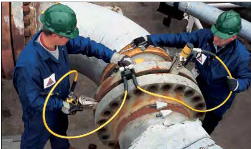
◀ Two FSH14 spreaders used simultaneously with Enerpac handpump, hoses and AM21 control manifold.
