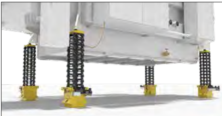
▼ Typical set-up with 4 Self-Locking Cube Jack and cribbing blocks to lift a transformer (hydraulic power pack and hoses not shown).
